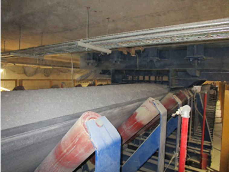
Image 1: Feeder conveyor during material discharge
