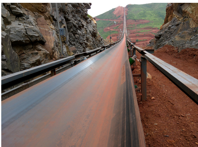
Figure 2. Blasting and excavating were required for creating a suitable route through the hilly region of the conveyor path.
