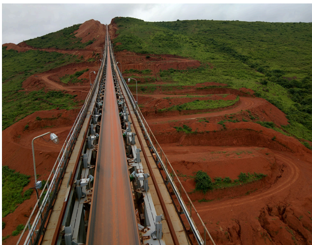
Figure 1. A very undulating terrain typified the path of the conveyor moving bauxite ore from the mine to the Utkal Alumina plant.
